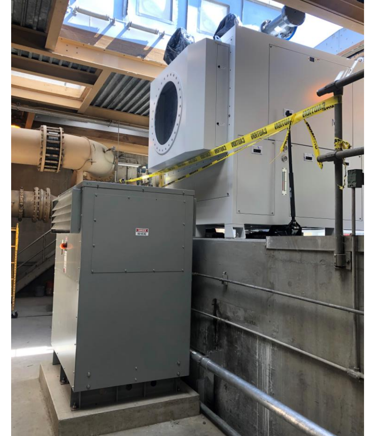
New APG Neuros Blower and Transformer
