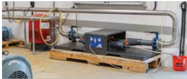
Moleaer's nanobubble generator was easily installed with little to no downtime for the wastewater plant.
