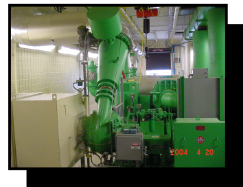
A single blower installed at Janesville, WI Utility replaces 3 older blowers and saves over $30,000 per year on their
